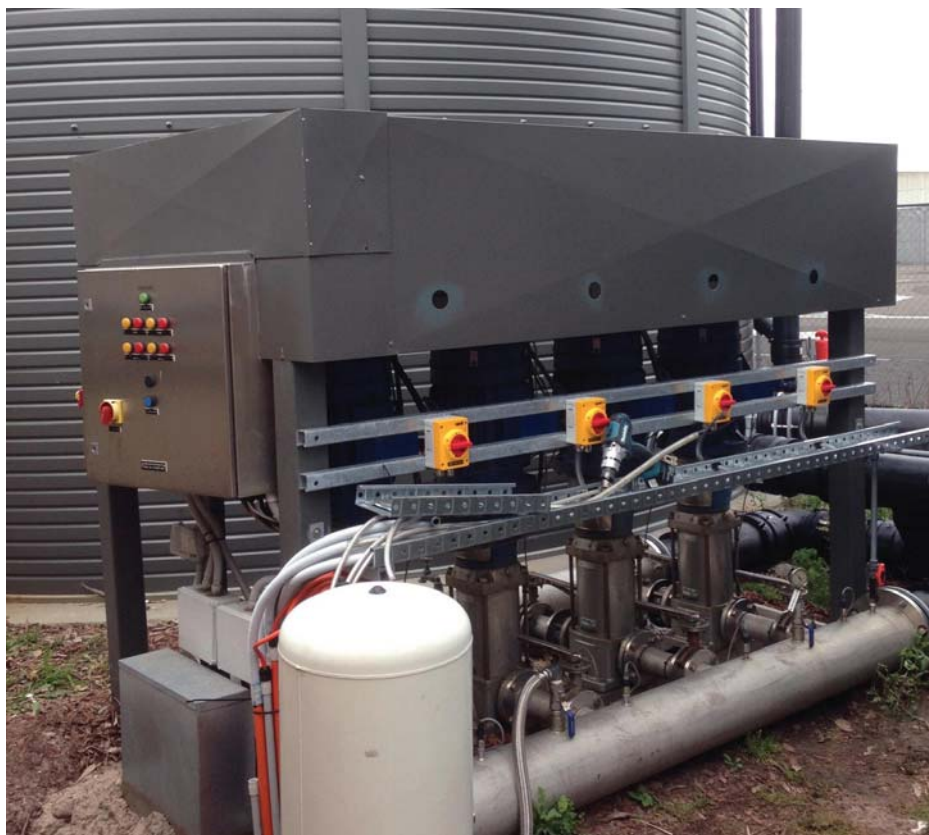
KATKO EMC safety switches installed to a water purification system at the Sydney International Airport.
